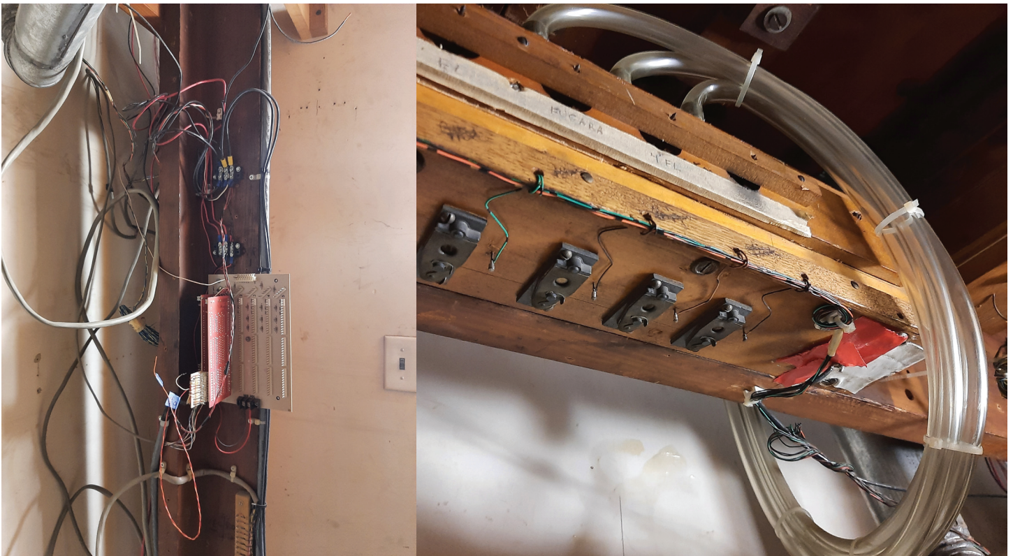
(below right) Damaged and poorly repaired stop action.
